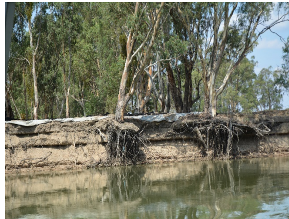
Murray River erosion (Barham 1.5 hrs drive) downstream of Barmah Choke
